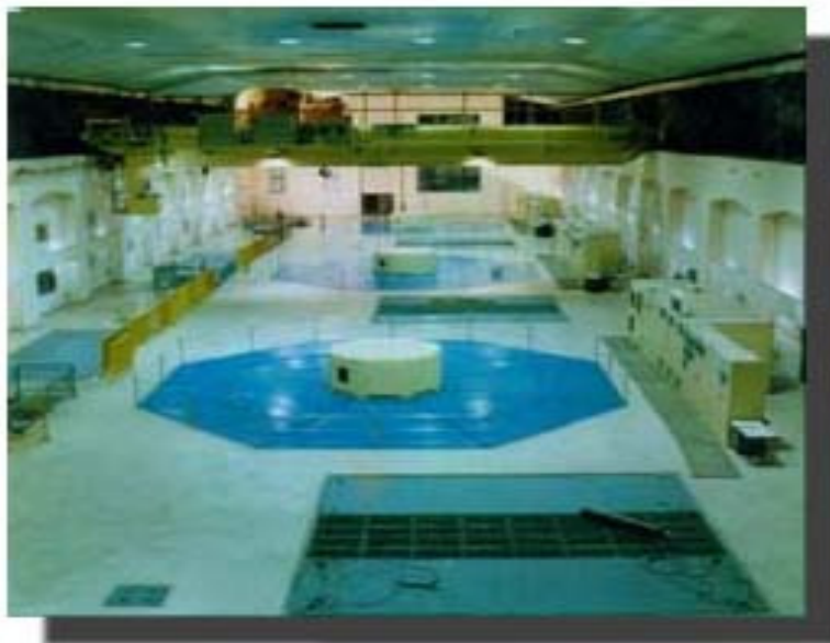
Figure 16: Chamera Stage - I Power Station (540MW), Operated by NHPC.
