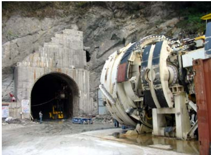
Figure 15: Parbati Stage - II Power Station (800MW), Operated by NHPC.
